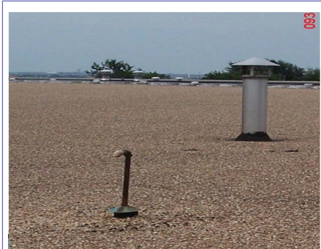
Figure 9: Safety valve piping outlets
