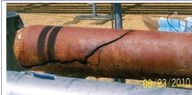
Figure 13: Liquid hammer can destroy even a heavy-duty seamless steel pipe
