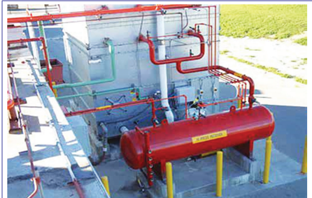
Figure 3: Piping showing all welded joints
