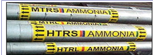
Figure 16: Pipe labeling as per the standard
