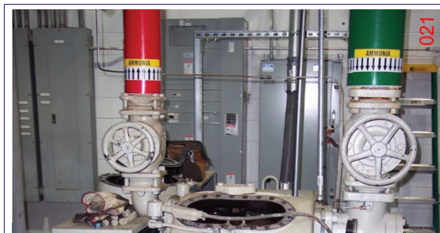
Figure 16: Pipe labeling as per the standard
