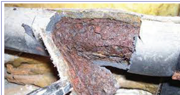
Figure 15: Corrosion under insulation (CUI) by conducting spot checks
